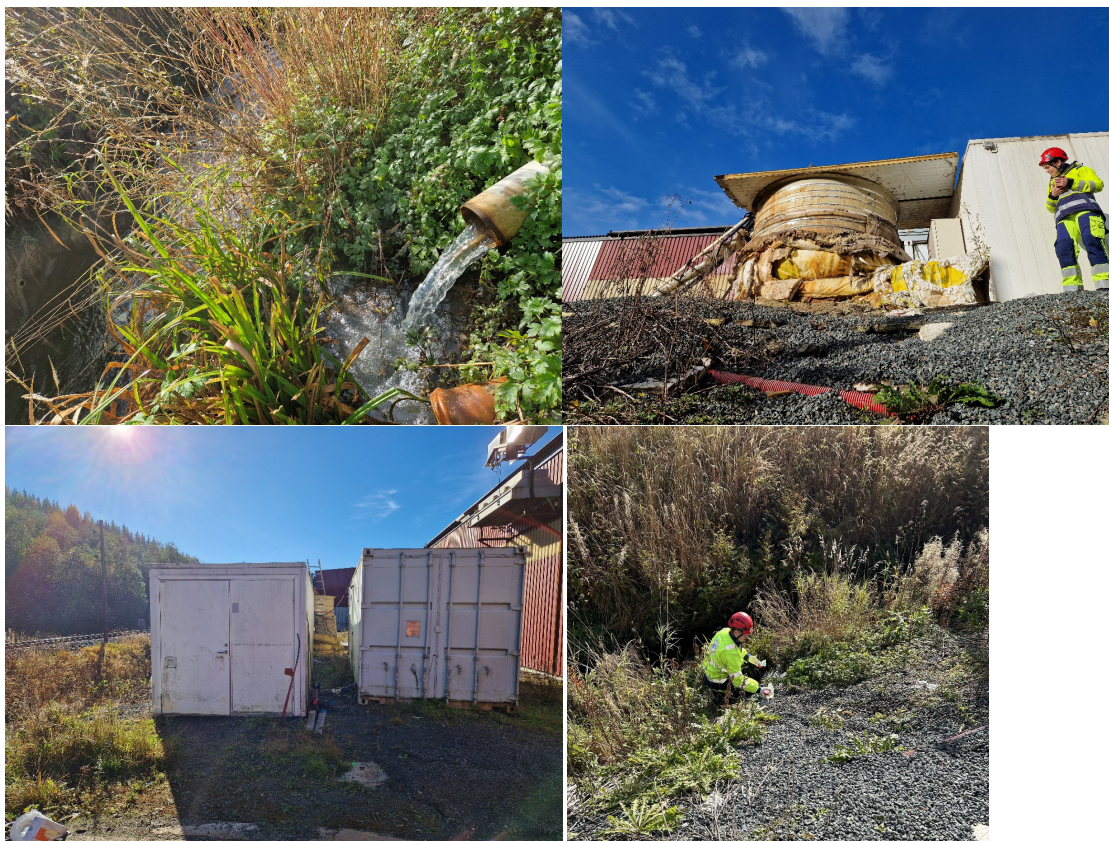
Figure 16: Treatment facility and sampling point for discharge of treated stormwater to the recipient.
